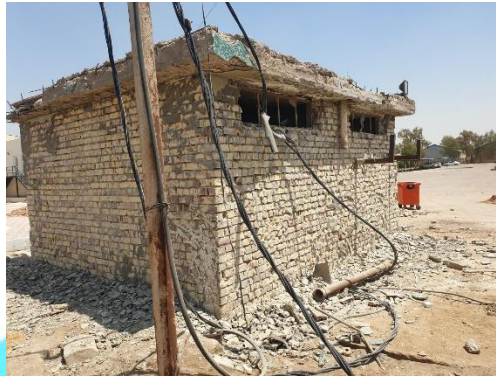
Installing 1.5m garden lighting poles on the sides of the students' .14 walkways.
